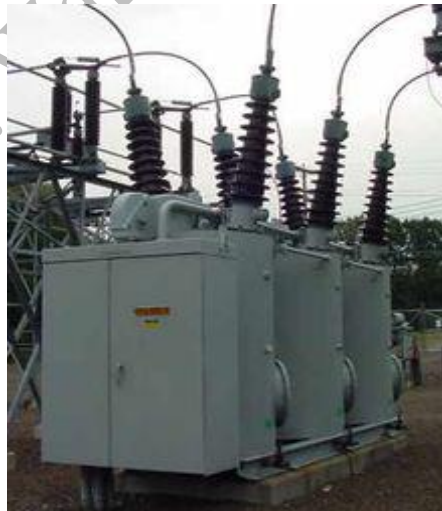
115 kV bulk oil circuit breaker
