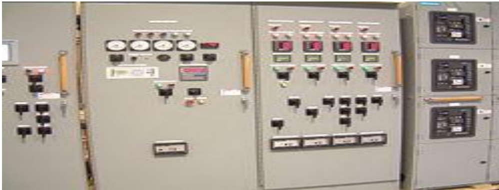
Fig.1.2 A section of a large switchgear panel, in this case, used to control on-board casino boat power generation.
