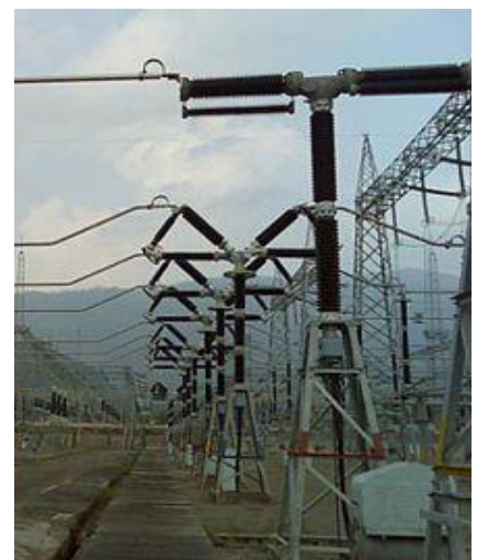
400 kV SF 6 live tank circuit breakers
