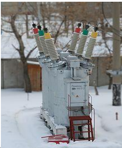
Fig.1.3- 110 kV oil circuit breaker
